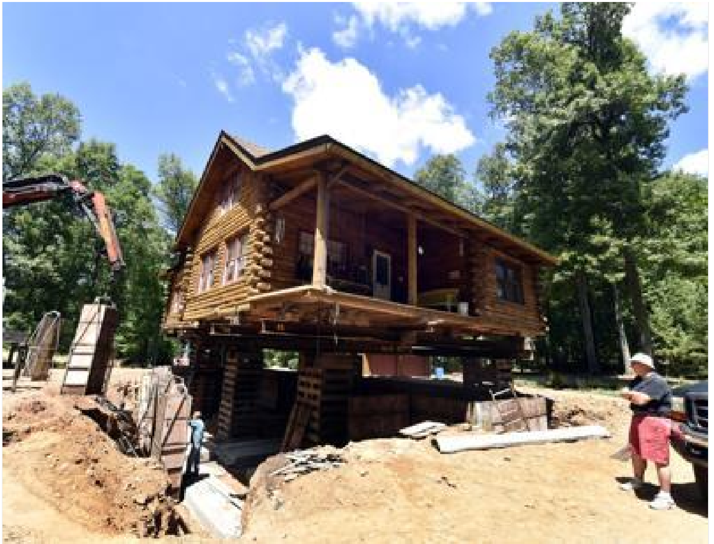
State Bond Commission authorizes next $20M for crumbling foundations
